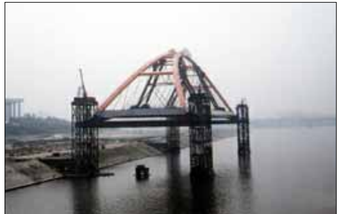
Above: Stage Two - raising the arch. From four lift points, one on each pier, Fagioli PSC L600 jacks perform a synchronised lift of the arch to a position where the barge and grillage can come underneath.
