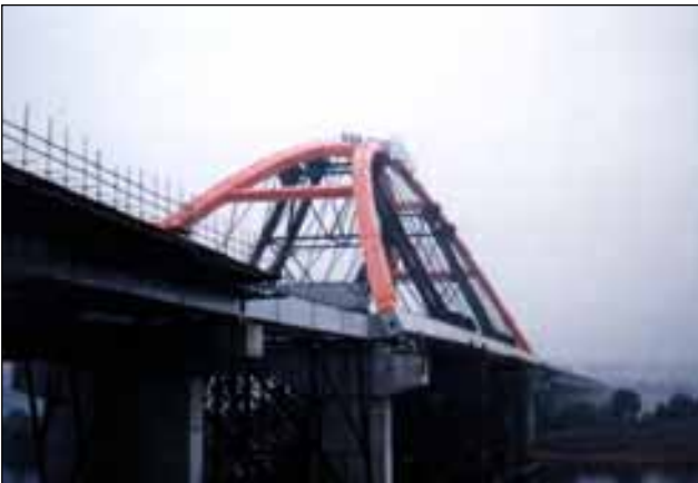
Above: The final positioning of the arch, not in Fagioli PSC's scope, was to tow the barge between the bridge piers and by ballasting down, the arch was placed onto its permanent bearings.
