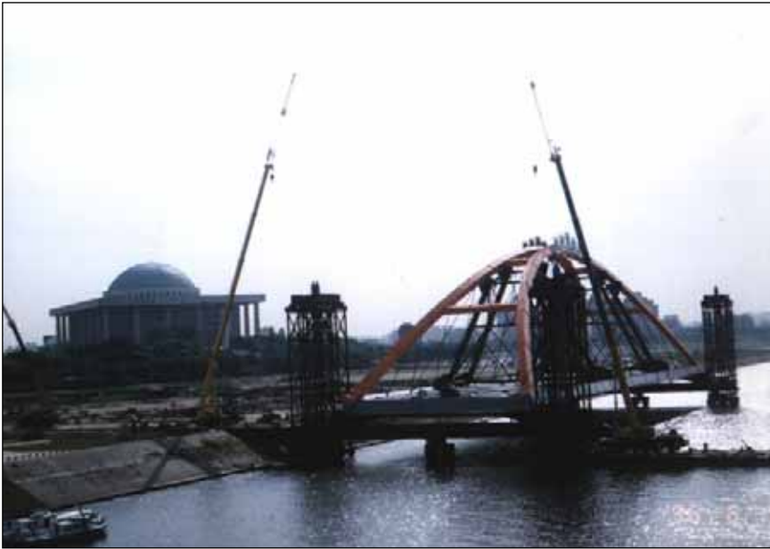
Above: Stage One - completion of the skid onto the finger piers. The skid track runs directly from the fabrication area, across extension pieces and onto the pier structure.
