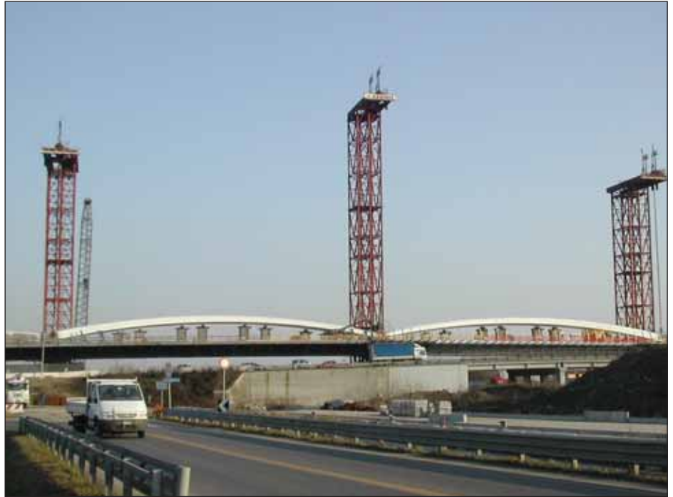
Above: Start of the lifting operation. Note temporary pin joint in centre of arch
