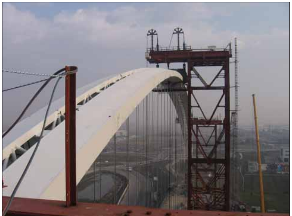
Below: Views from one of the side towers to the centre tower. Note cantilever jack support arrangement for the two L180 jacks
