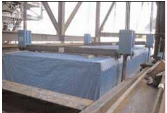
Below: Close up of the fixed anchor units attached to the generator.
