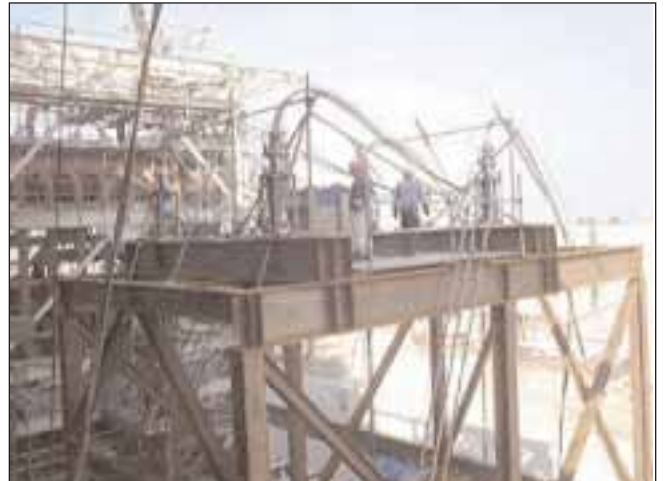
Above: Close up of the travelling frame with the strand jacks on top.
