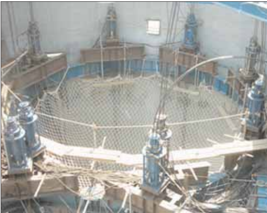
Below: Arrangement of jacks and jack supports at top of the structure
