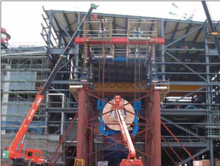
Above: Lifting of 360 MT Gas Turbine by six L100 jacks to a height of 12 metres.
