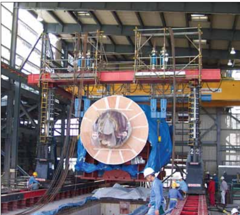
Below: Gas turbine moving to its final location by lift & lock hydraulic gantry.
